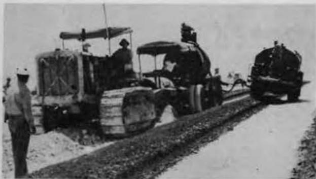
WINDROWS of coral being mixed in place in the process of surfacing a runway.
