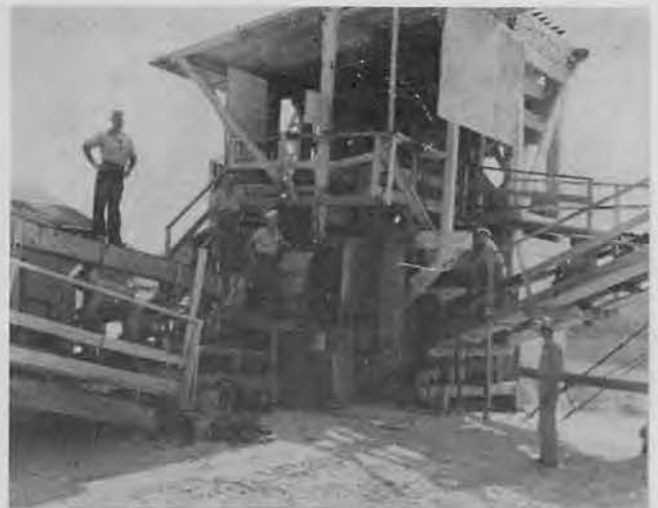
Morsette, Reeder, Spence, Rickard, Chiarello and Lt. (jg) Bett at aggregate plant crusher.
