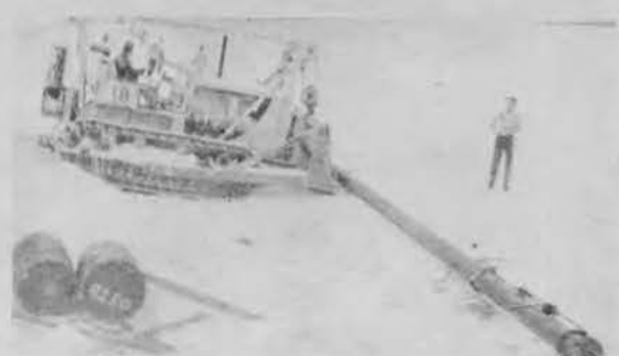
A 200 foot section of pipe fabricated on the beach, about to be launched and floated into position.
