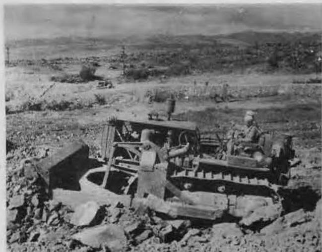
CLEARING A SITE for more barracks, one of our dozers pushes around some of Oahu's volcanic rock.
