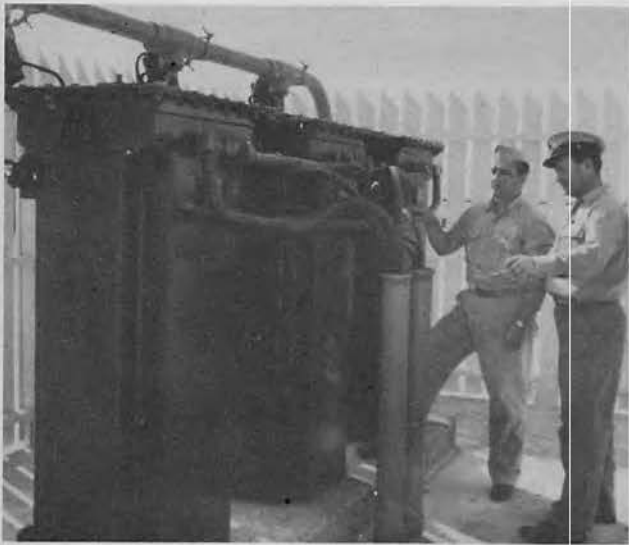
ELECTRICAL WIZARDS Vose and Donnelly admiring a neat transformer bank of their creation.
