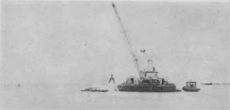
There are faster ways of dredging a channel, but Gildy's crews made over 800 yards a day with this rig.
