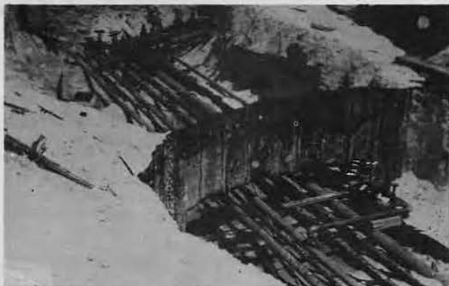
WITH ALL SERVICES in the same trench, our pipefitters had to have their wits about them or end up with salt water in the lube oil.
