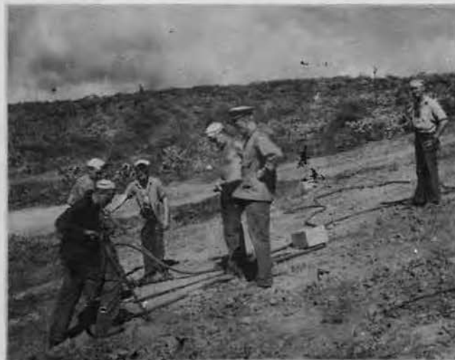
DYNAMITERS making it easier for the bulldozers by blasting away portions of a hill.
