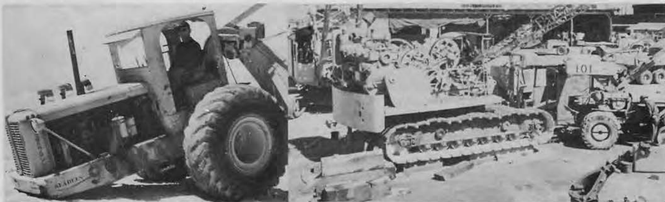
KNAPP'S TIRED TURNAPULL. These giant earthmovers carried 14 yards of coral each trip, at 20 miles per hour. FACILITIES FOR COMPLETE OVERHAUL of all heavy equipment were maintained by the Battalion.
