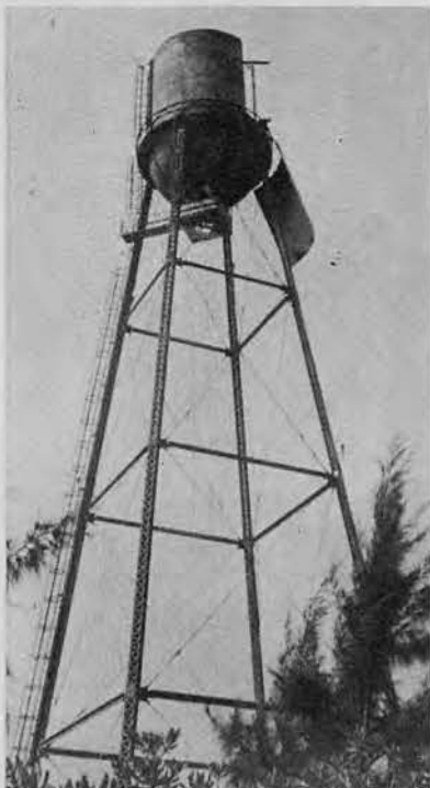
REMOVING the tank from the tower preliminary to moving it to a new location.
