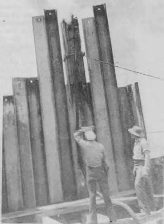
PILE HAMMER making its own clouds as two sheet piling are driven to grade.
