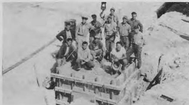
CHIEF DONOVAN'S manhole builders apply a loadtest to their framework—or are they just posing?
