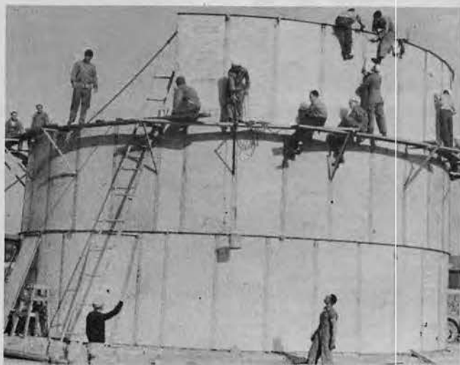
CHIEF THOMPSON AND CREW missed some hikes at Camp Parks to build this 10,000 barrel bolted steel tank.
