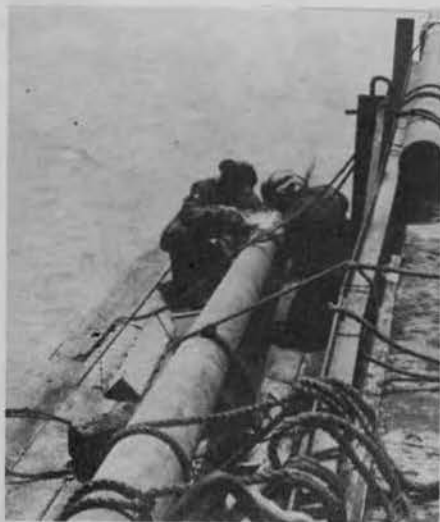
Welders had to be good sailors to repair the breaks in this large fuel line.
